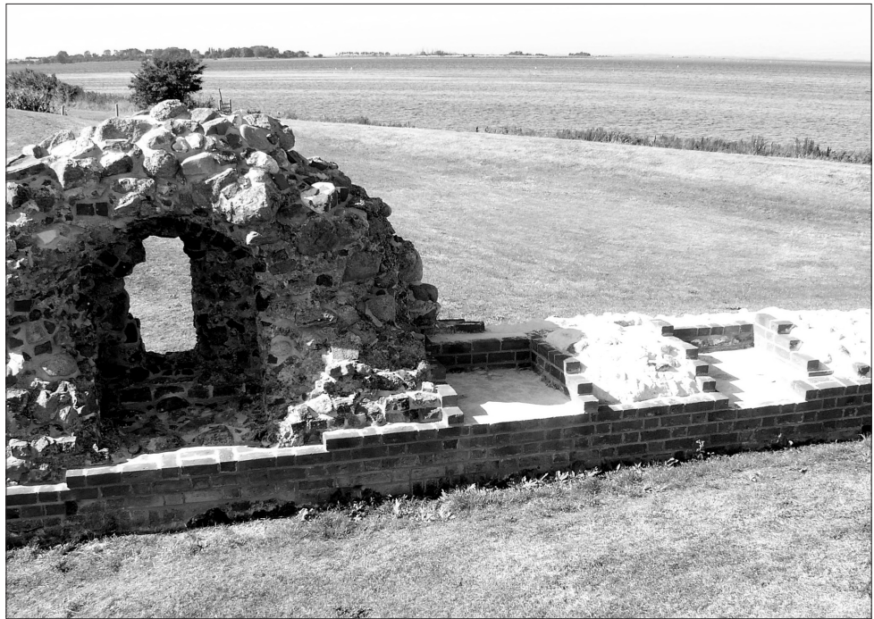
Fig. 15. Canon loops in the western flanking wall after repairs. The original, high wall core has been waterproofed. New medieval-style bricks have been laid on the facades of the flanking walls and in the poorly preserved canon-loops. The new bricks have been placed in accordance with reliable traces in the mortar. Photo: J. Frandsen, The National Museum.
